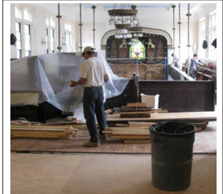
Garbade Room under construction. Note that the floor is now level with the rest of the balcony floor.
