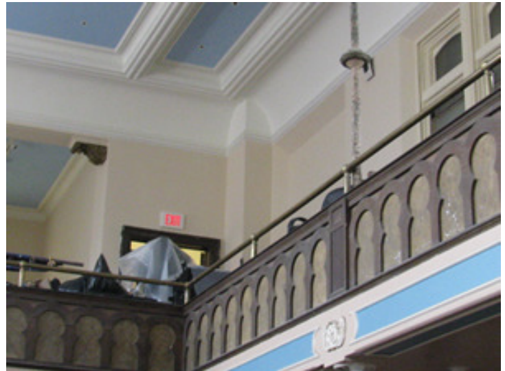
Repaired plaster and a first coat of paint in the balcony (June 25)
